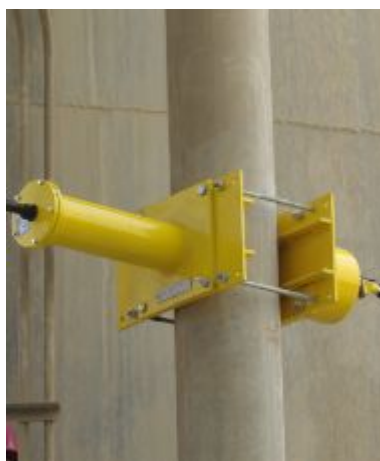
AM/KM-825探测器及射源现场安装图
